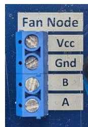
Figure 6: Termination Points on the EPIQ Cable Node for connection to the EPIQ+ Fan Node
